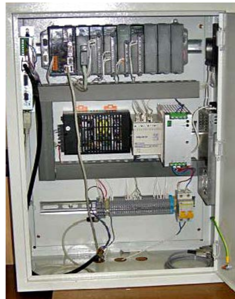
Device control panel
